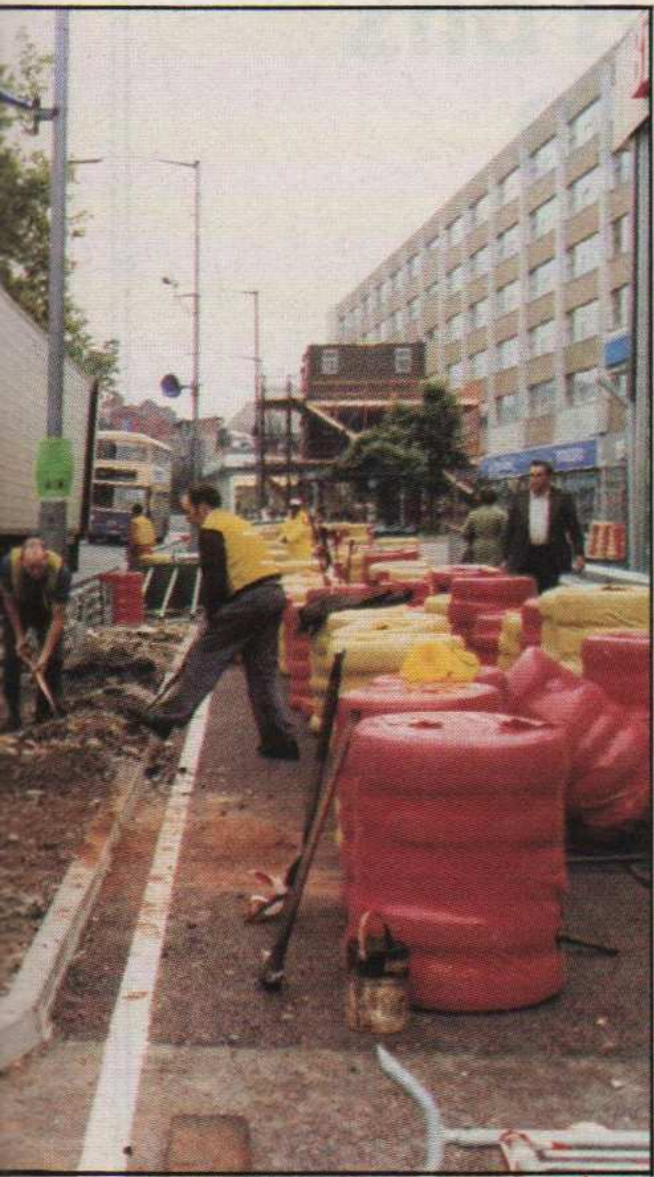
Council workmen erect eight miles of steel 'armco' barriers around the course while each nut and bolt is checked by international motor racing officials before racing can start. Two rail and even three rail barriers are used to border the track each side while stacks of bound tyres are also used to absorb impact of any wayward cars, the Birmingham streets taking on a Monaco appearance.
